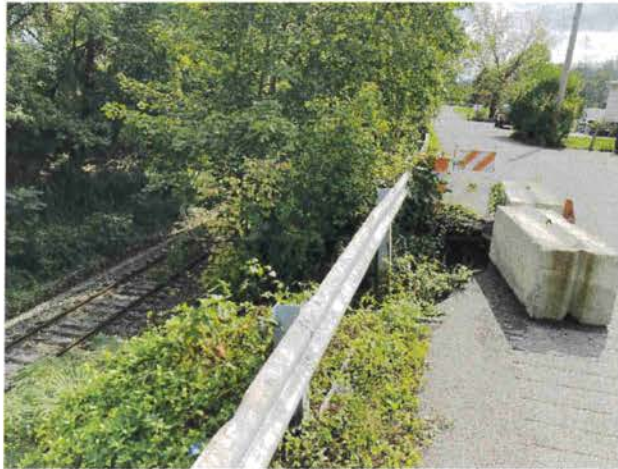
Current landslides on Werner St.
