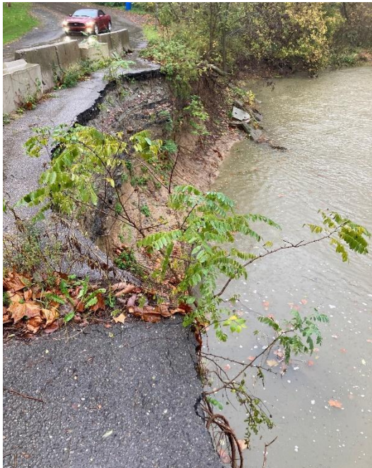
Photo of Before Conditions:
