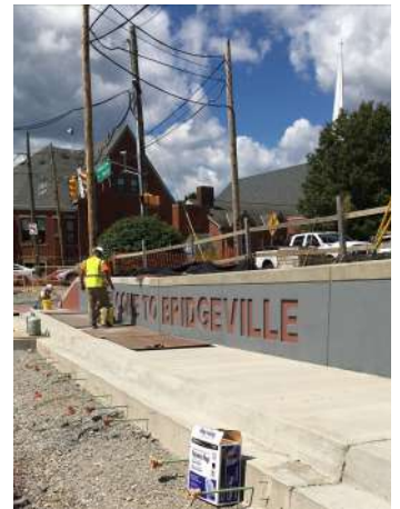
Welcome to Bridgeville wall built as part of the Chartiers Street Widening
