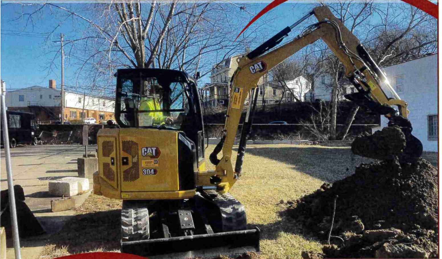
New Public Works Excavator working to install water service for the Baldwin Street Pollinator Garden.
