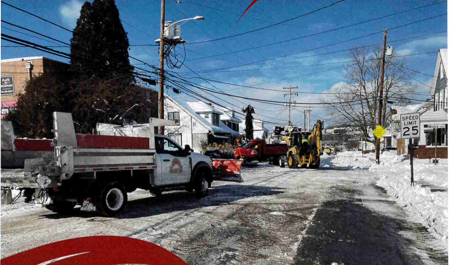
Public Works Dept removing large snow piles from Hickman Street following the January 25th Snowstorm that covered Bridgeville with over 12" of snow.
